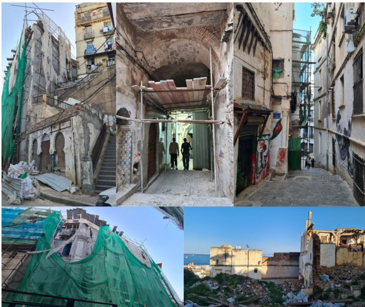
Fig. 10. Deterioration of the buildings of the Casbah. Source: taken by the author.
